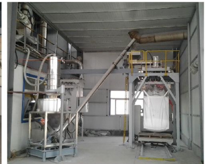
CHEMICAL PACKING MACHINE LINE
