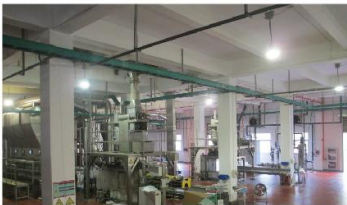
CHEMICAL PACKING MACHINE LINE
